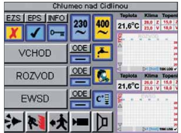
Control panel of remote unit
